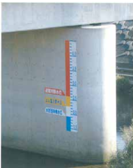
Example: Staff gauge for hazard
